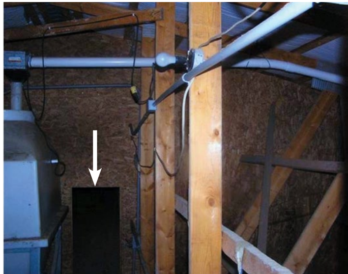
Figure 3.7. This attic fire stop has an opening cut into it (arrow), removing its effectiveness in containing a fire.
