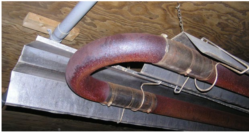
Figure 1.5. Radiant tube heater lacking heat shield. Note close proximity to combustibles (wood ceiling and conduit). (Photo credit: R. Drysdale, Farm Mutual Reinsurance Plan)
