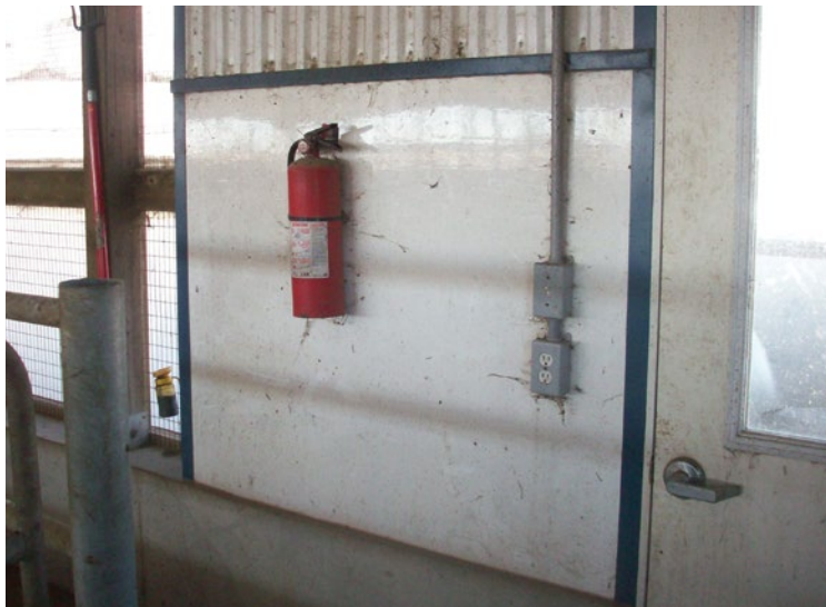
Figure 4.1. A fire extinguisher located next to an exit.
