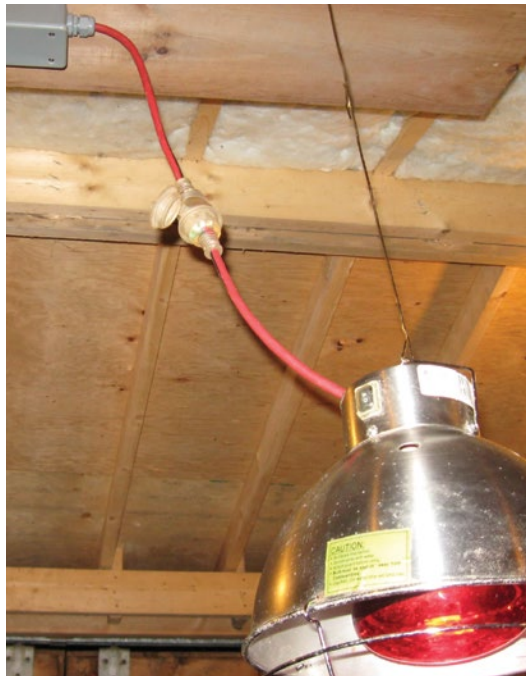
Figure 3.13. The heat lamp is connected directly to a wet-rated electrical box and includes a wet-rated cord cap connection so the lamp fixture can be removed. When the lamp is removed, the cover is placed on the female cap end to protect it from corrosion.
