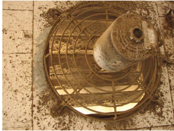
Figure 2.7. Example of a dirty fan in need of cleaning.
