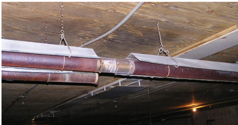
Figure 1.4. Radiant tube heater with heat shield displaced. Note charring on the ceiling.
