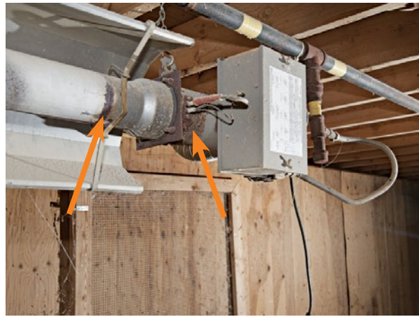
Figure 2.8b. Front view of a radiant tube heater inside the same broiler barn. Corrosion is present.
